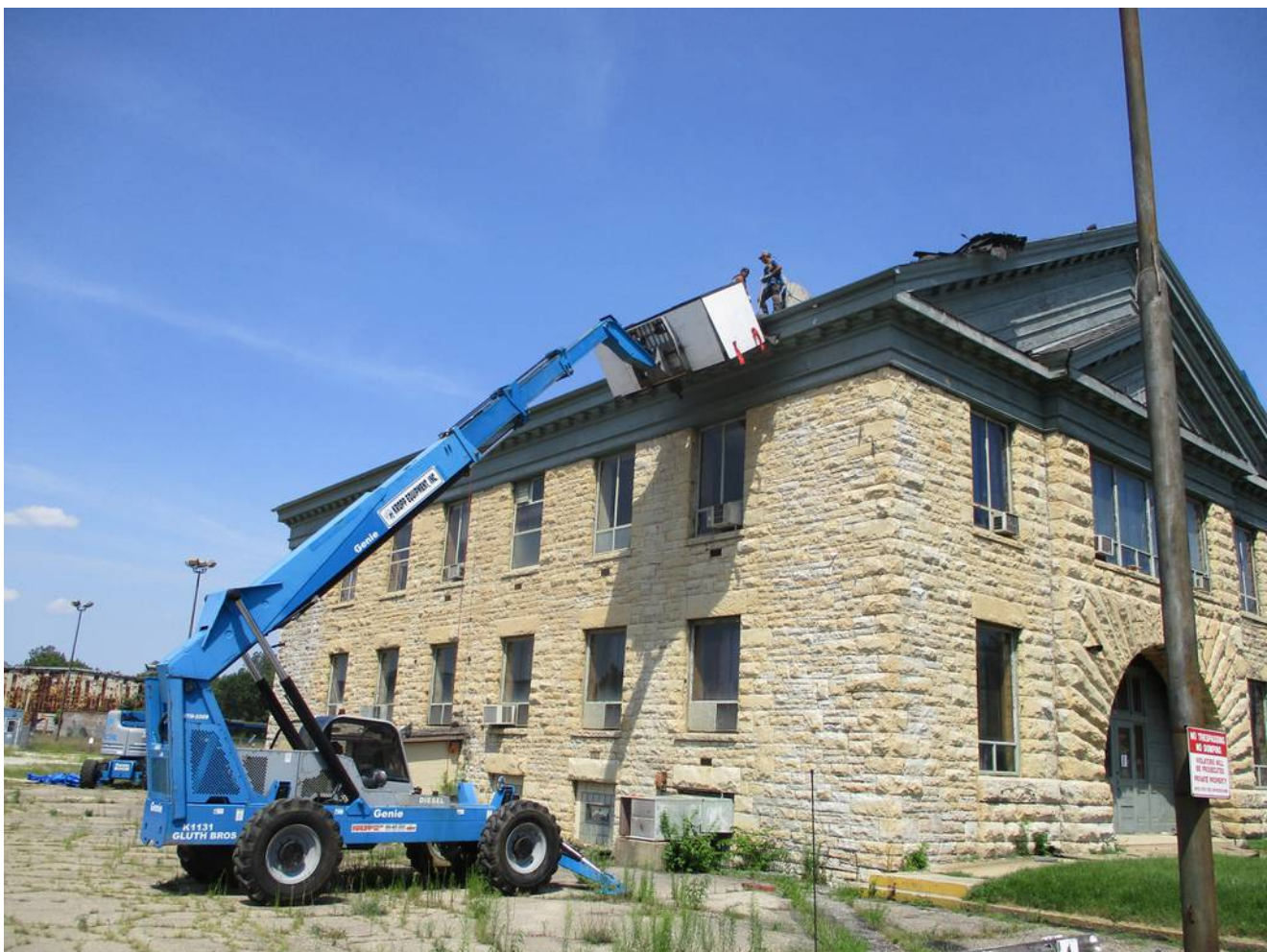
Repairs to the roof of the vacant main office building at U.S. Steel were made in 2021. (Bob Okon)
