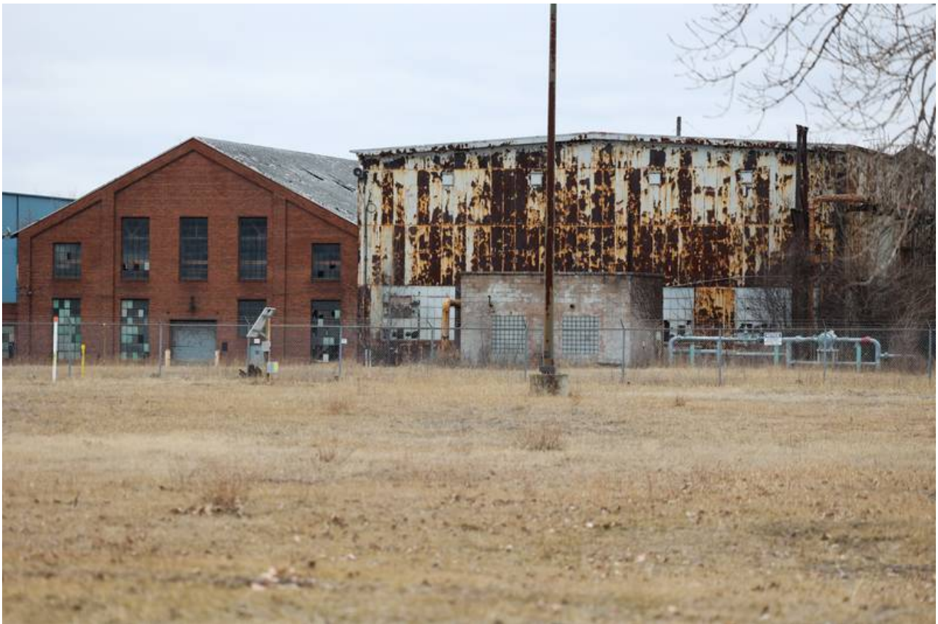
Buildings at former U.S. Steel site continue to deteriorate along Collins Street in Joliet. (Gary Middendorf/Gary Middendorf)
