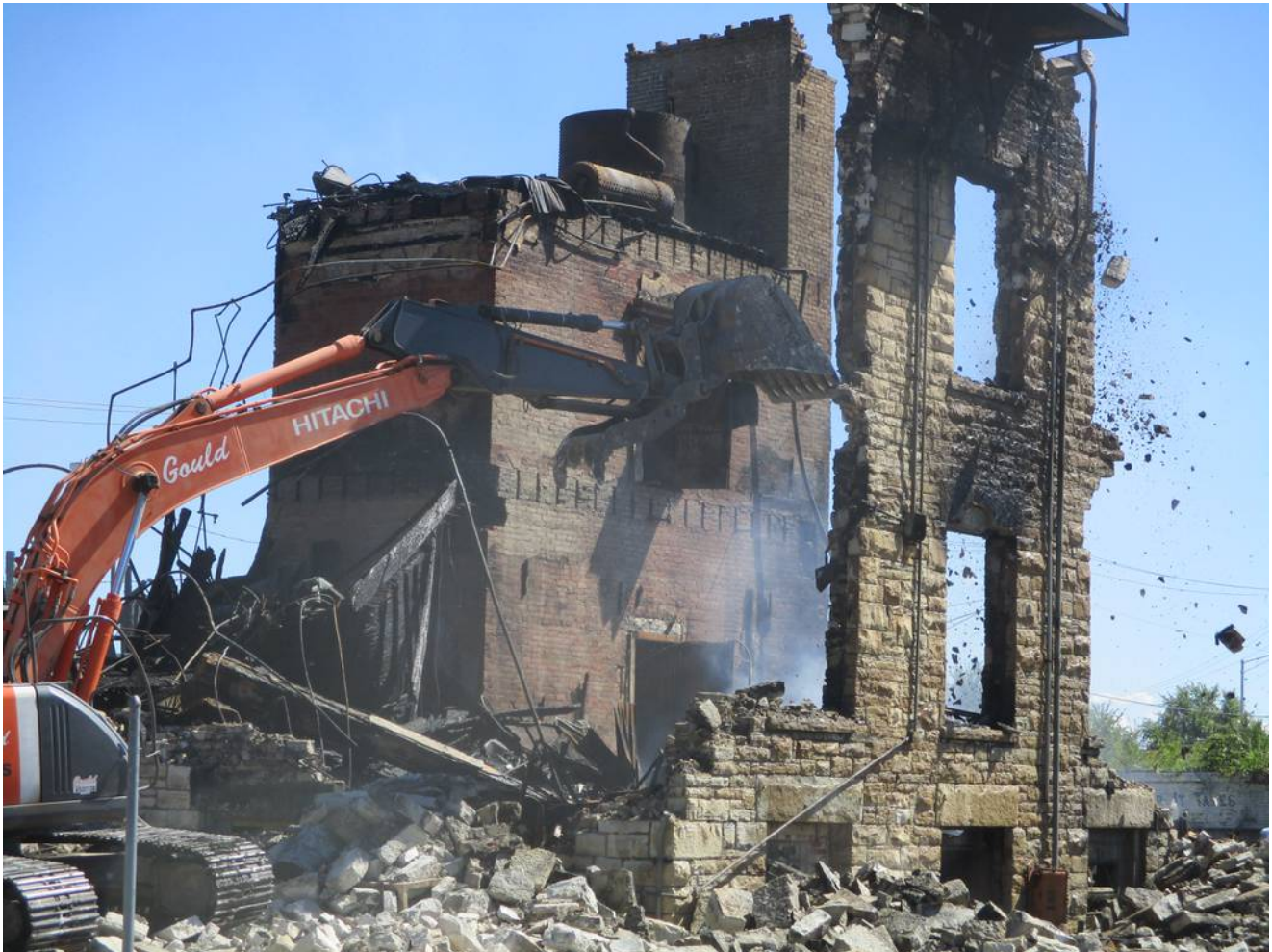
A wrecking machine on Saturday tears down the limestone exterior of the old U.S. Steel Main Office Building at 927 Collins St. in Joliet after a devastating fire that was reported at 3:11 a.m. Sept. 7, 2024 (Bob Okon)
