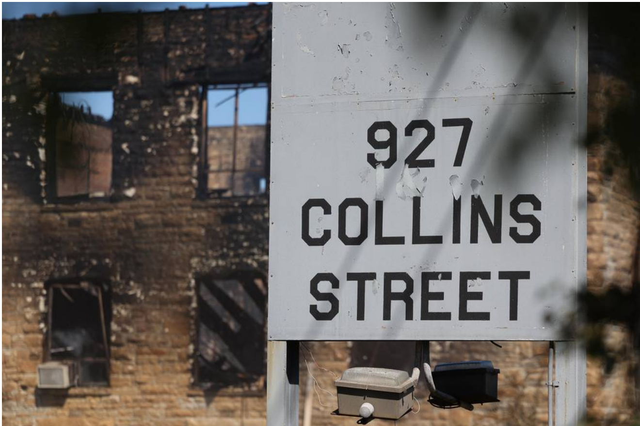
Only the brick walls remain standing at the historic U.S. Steel office building after a fire on Saturday, Sept. 7, 2024 in Joliet. The historic building along Collins Street was engulfed in flames early Saturday. (Gary Middendorf)
